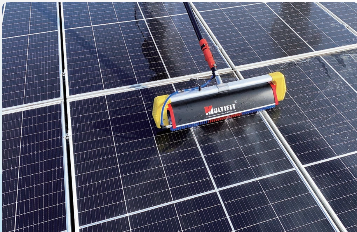
MULR-D Pro on factory rooftop system
